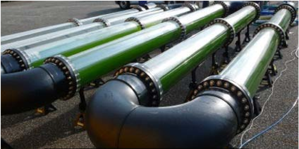
South Australian R&D Institute – Photo Bioreactor
