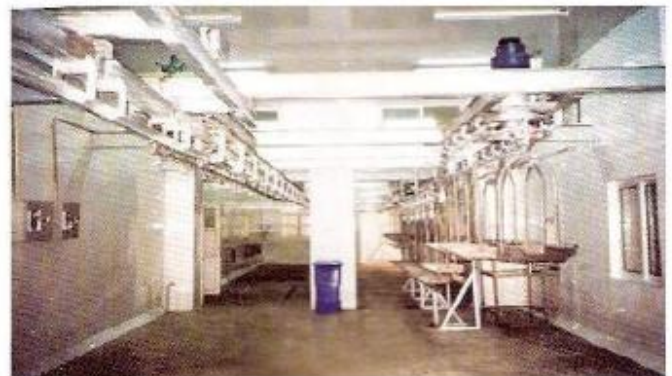
Hanging-type Dissecting Pushing Line & Inner Viscera-Inspection Conveyor
